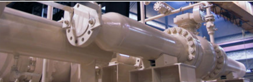
Skid Mounted Pipe Spools
